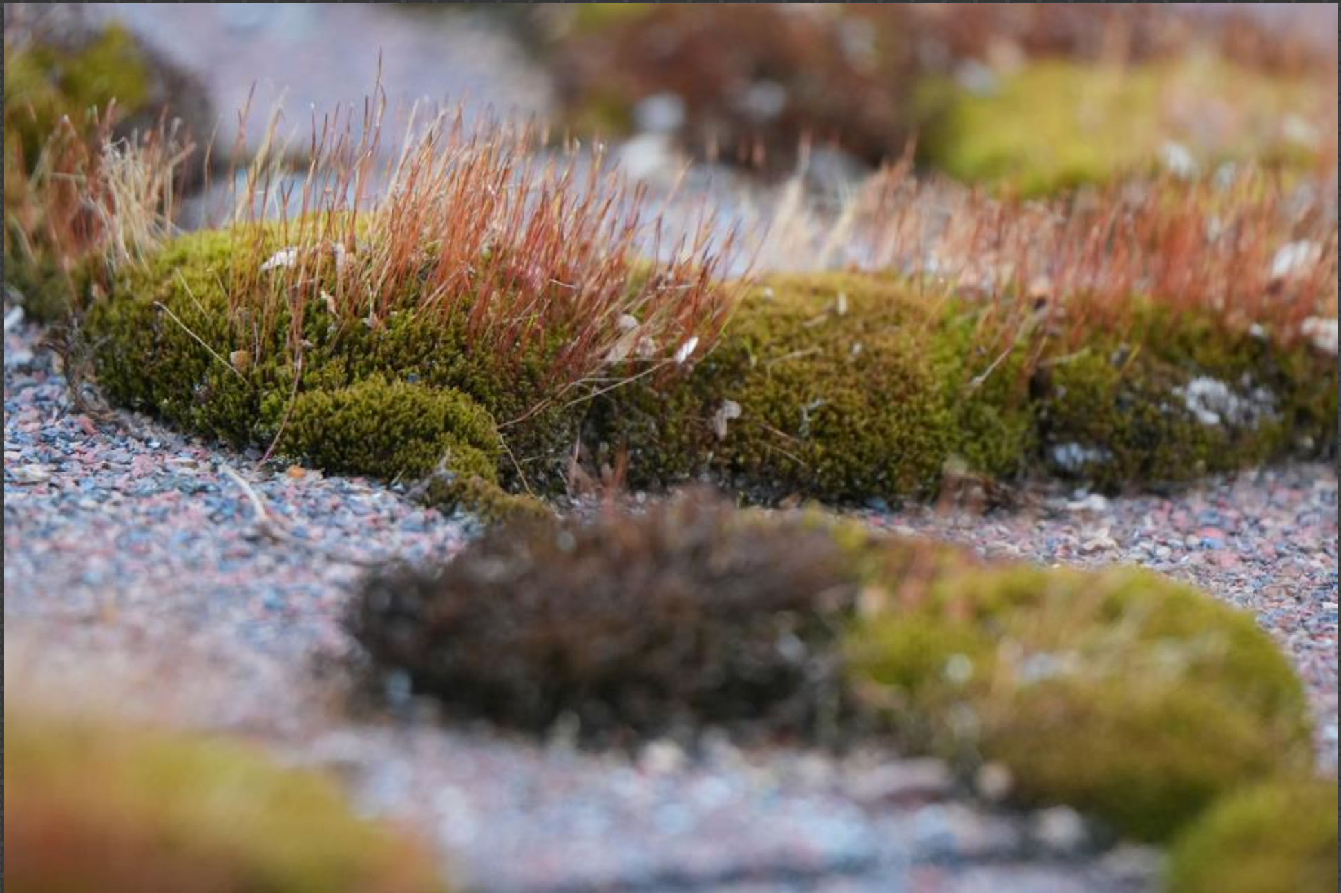
603-ADW – Moss on Shed Roof
