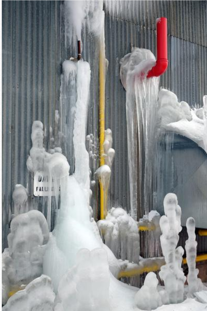
10-Gary Benson - Western Insulfoam Danger Falling Ice
